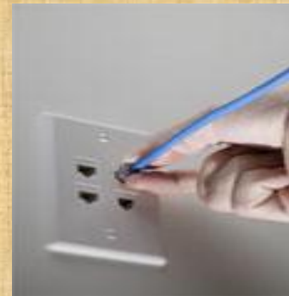
Wall Data Port
